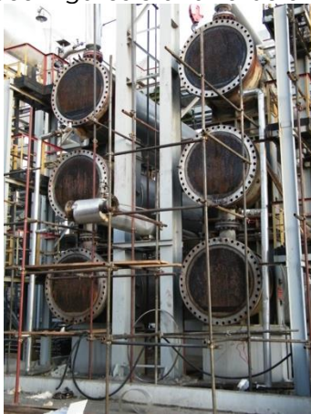
Figure 9: six shell exchanger, 30,000 tubes, partial condensation on the tubeside. Courtesy of Lukoil, Russia
